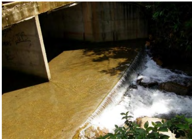
FIGURE 2 A box culvert with a smooth concrete bottom that accelerates streamflow and forms a waterfall that is a barrier to some small animals or fish.
