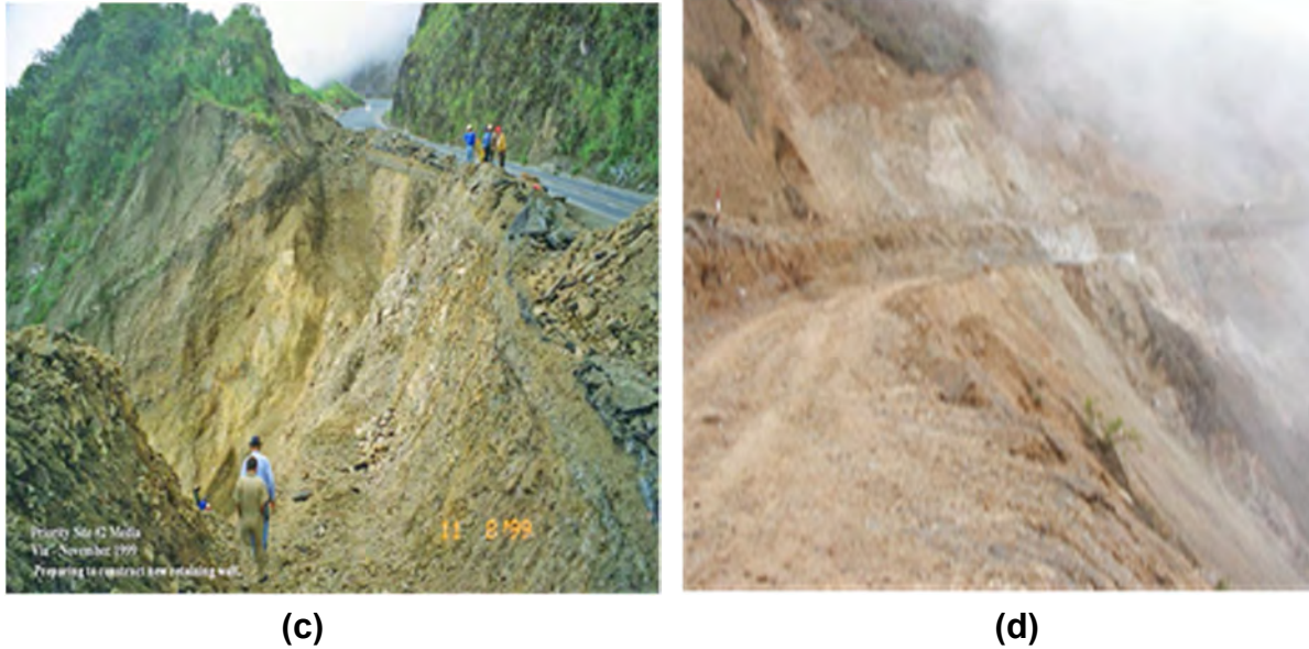
FIGURE 1 (continued) (c) Typical slope failure of approximately 25 \cdot 10^5 \text{ M}^3 ; and (d) Typical slope failure of approximately 25 \cdot 10^5 \text{ M}^3 . Notes: The photos present the general locations and typical slope failures along the Ecuadorian C-M-E mountainous LVR taken on November 1999, after the end of the Ecuadorian Andean 1998 El Niño flooding damages. Also, during this visit the road was already open following continuous road repair and maintenance activities, including clearing and removing of cohesive-granular and rocky slopes fallen materials.
