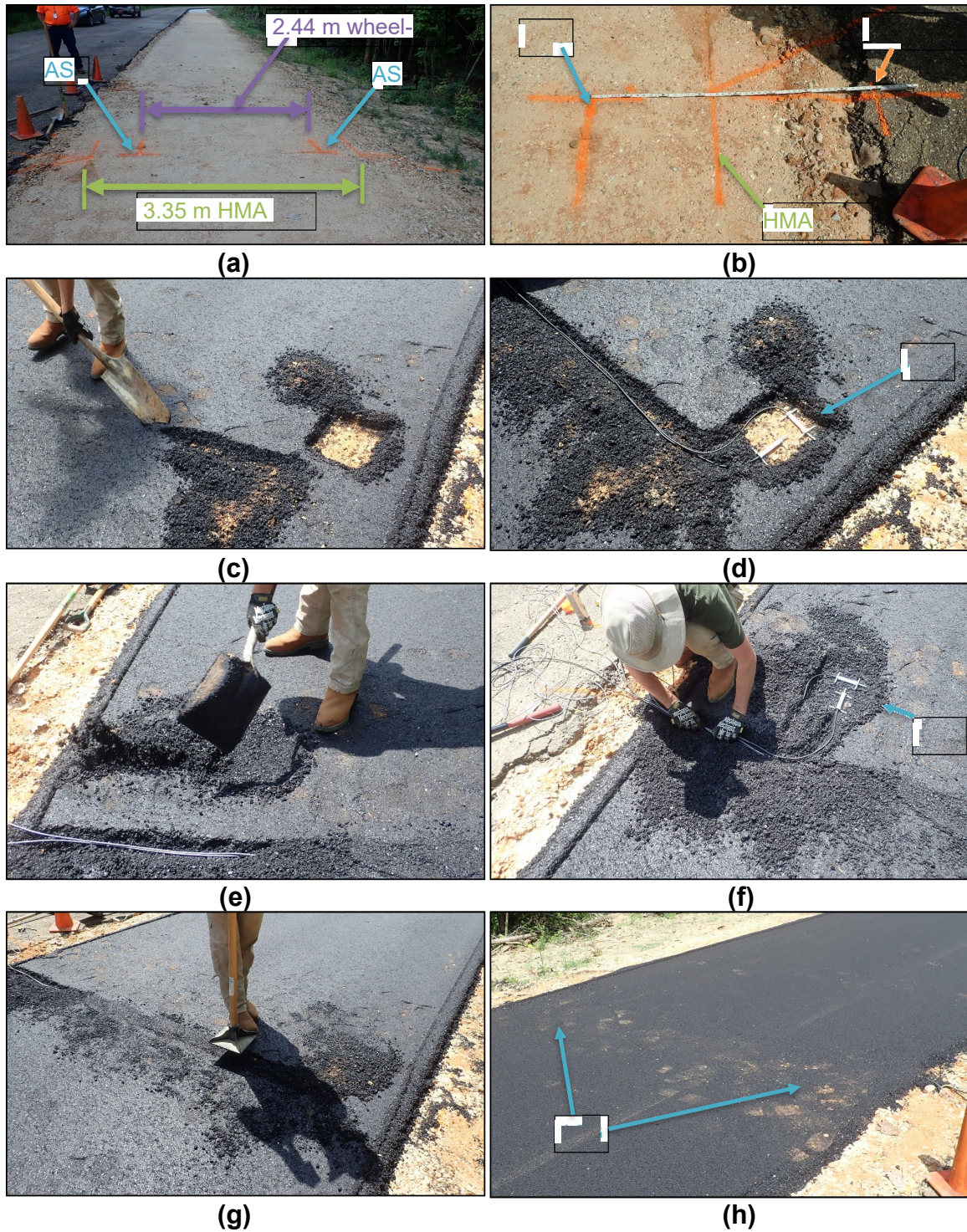
FIGURE 1 ASG installation: (a) ASG layout before paving; (b) establishing reference outside paving lane; (c) excavating HMA for ASG cabling; (d) ASG in place before backfilling, full depth; (e) excavating HMA for ASG; (f) ASG in place before backfilling, partial depth; (g) tamping backfilled HMA; and (h) final compacted HMA surface.
