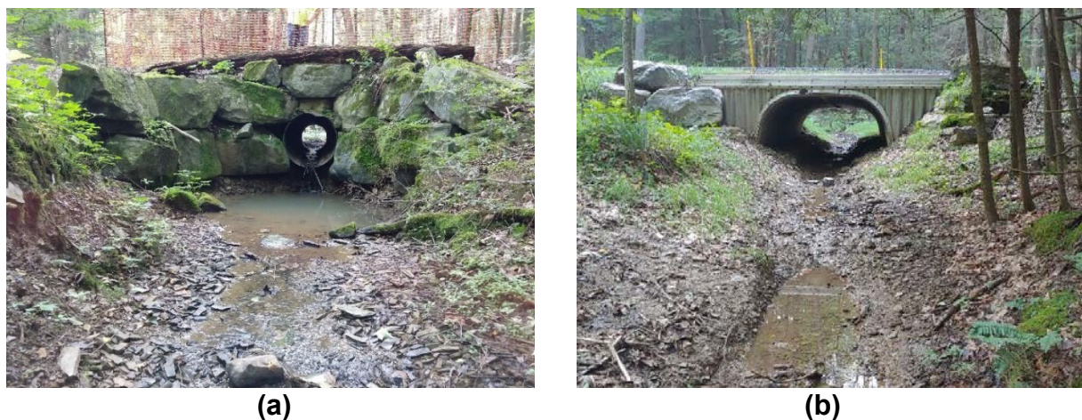
FIGURE 1 (a) Before and (b) after the replacement of a 3-ft corrugated pipe with an 11-ft bottomless structure. The existing pipe was constricting the 8-ft bankfull channel and caused large outlet drop and scour hole.
