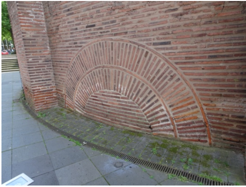
7.60 Bricked-up remnant of ancient heating system ( praefurnium ), seen on the building exterior. xiv
