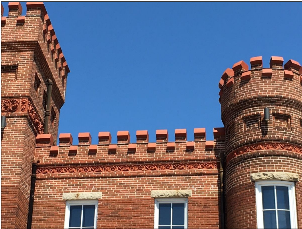
Figure 10. Tower and cornice details on the Leigh Street Armory. Source: Historic Richmond.
